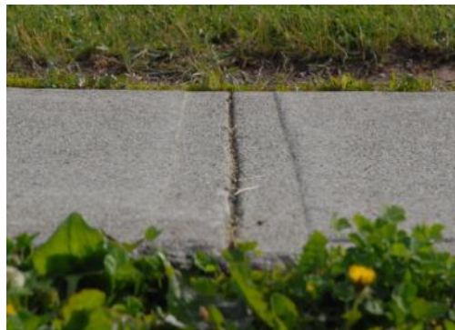
Bumpy Sidewalk surface with Tooled Contraction Joint
