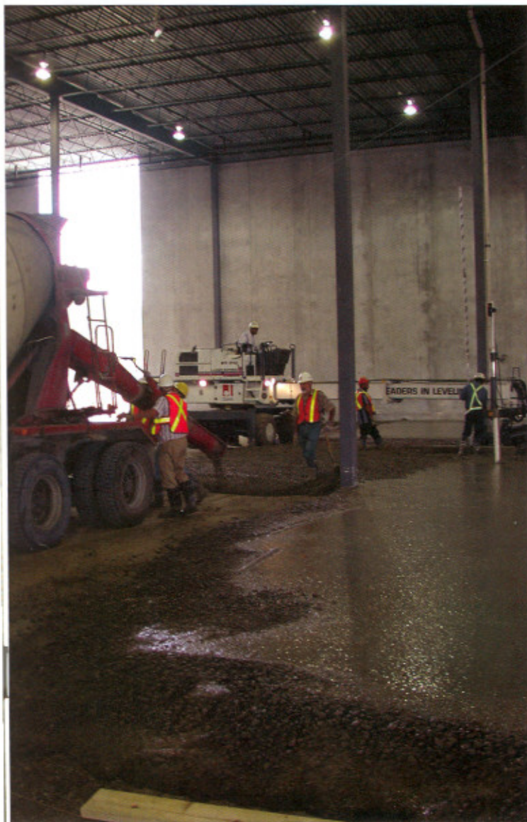
Achieving specified floor tolerances is a function of many concerns, including the quality of ambient conditions, the workability of concrete, and the selection and quality of methods of construction.
